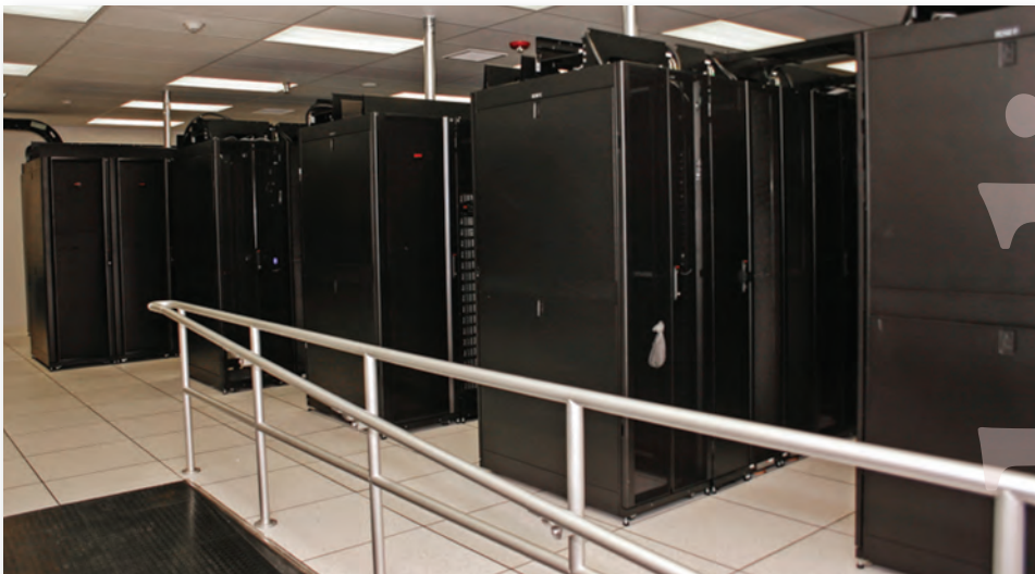
One of the ChimeNet co-location data centers.
