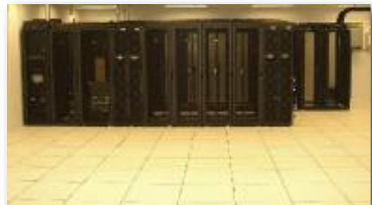
ChimeNet co-location data center
